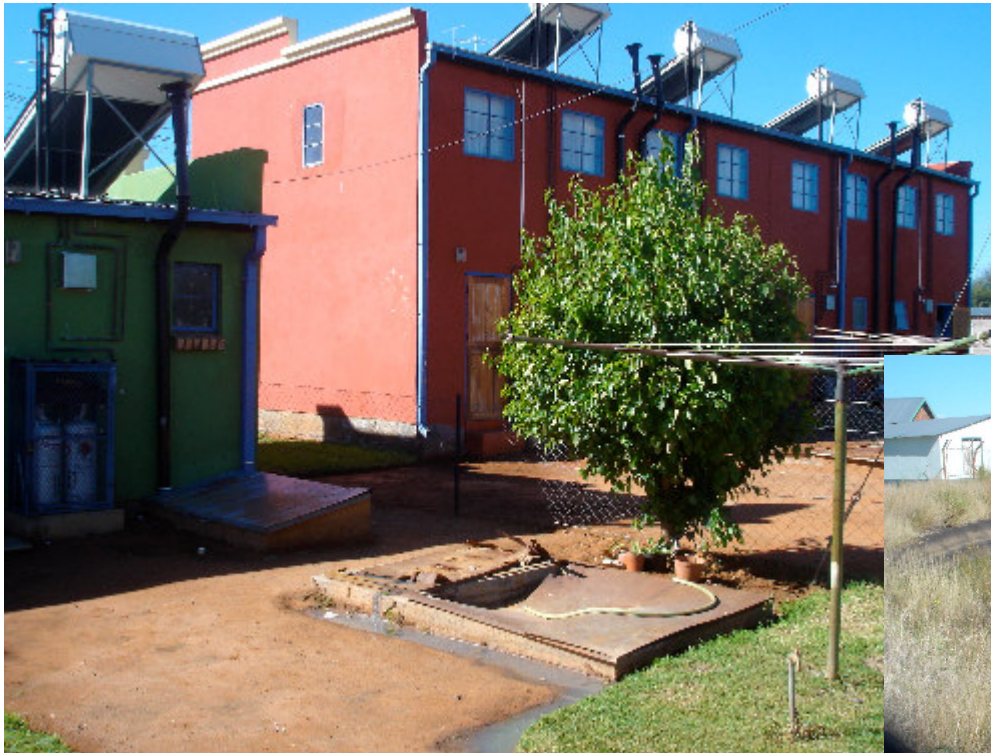
Clogging sandfilter and pond system in Moshoeshoe (Ecovillage), May 2006
